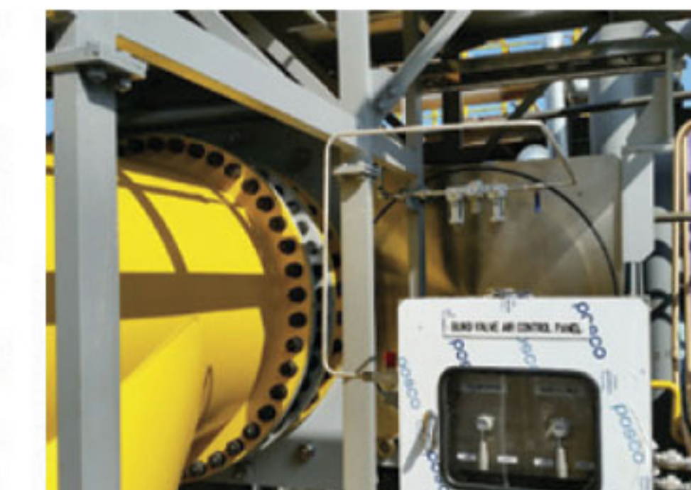
Coke Oven Gas(AOV automation)
