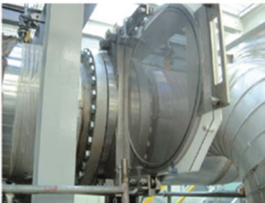
Heat Exchanger-Bypass Line
